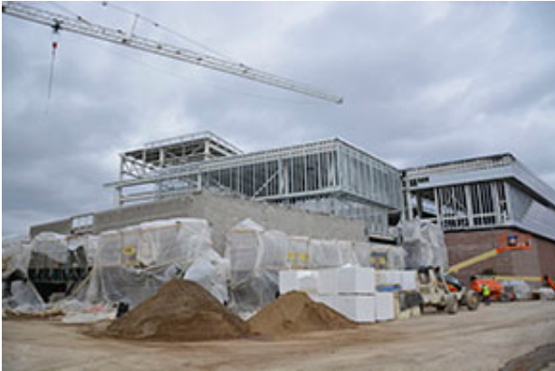
A view of the FRIB construction site. Civil construction is 10 weeks ahead of schedule.
