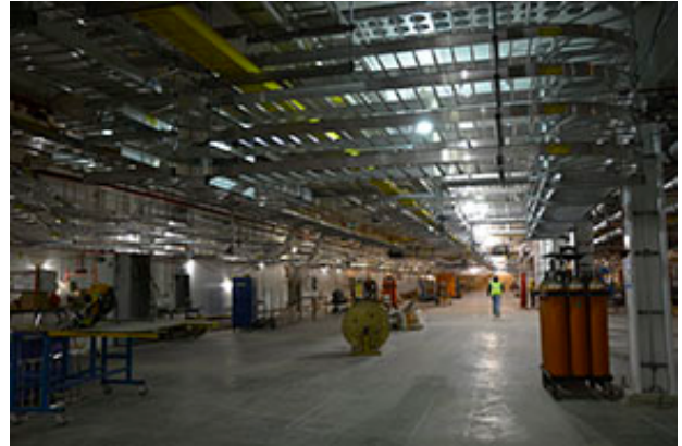
A view of the linac tunnel, one area where mechanical, electrical, and plumbing work is underway.
