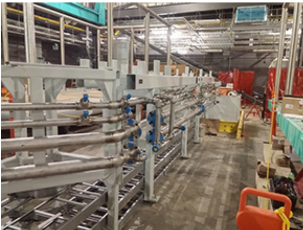
The Accelerator Systems Division installed front-end accelerator components early thanks to the Conventional Facilities and Infrastructure Division completing the front-end building ahead of schedule.
