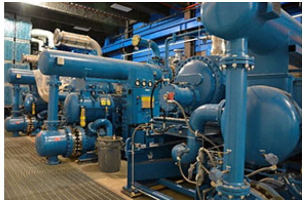
This photo shows three of six helium compressors installed in the FRIB construction site.
