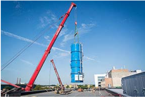
The 100,000-pound vertical cryogenic cold box arrived at FRIB on 10 August. The cold box was built in Oklahoma and arrived in Michigan by way of the Lake Michigan car ferry SS Badger.
