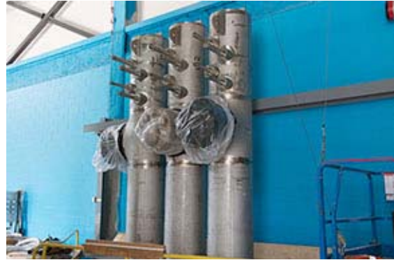
Using cranes, vertical cryogenic transfer lines were lowered into the cold box room through a roof hatch. Each of the three transfer lines will deliver liquid helium to a segment of the linear accelerator.
