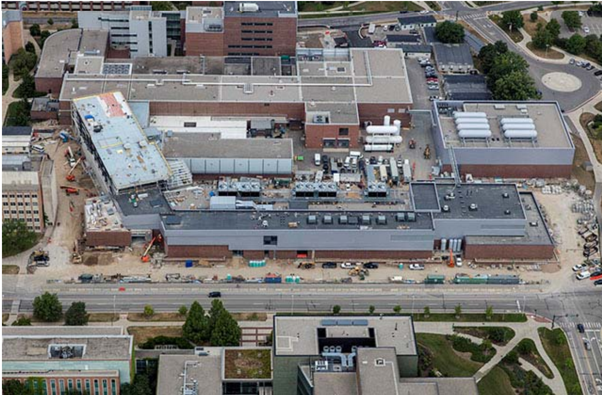
FRIB civil construction continues to progress 10 weeks ahead of schedule, with an increasing number of technical installations. This aerial shot of the construction site was taken 7 July 2016.
