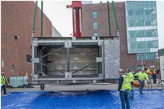
The 85,000-pound wedge vessel was delivered in October and is currently being tested. After testing, the wedge vessel will be installed in the target area.
