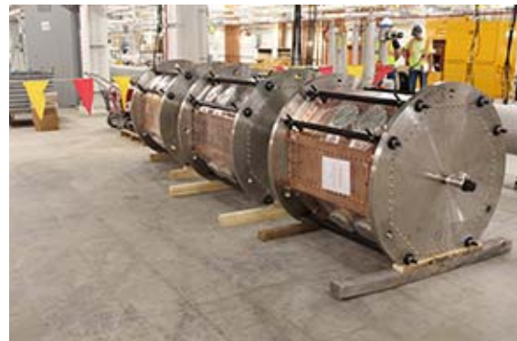
FRIB's Conventional Facilities and Infrastructure Division assisted in the placement of the radio frequency quadrupole (RFQ), which weighed approximately 30 tons. The RFQ will prepare the beam for acceleration in FRIB's superconducting linear accelerator.
