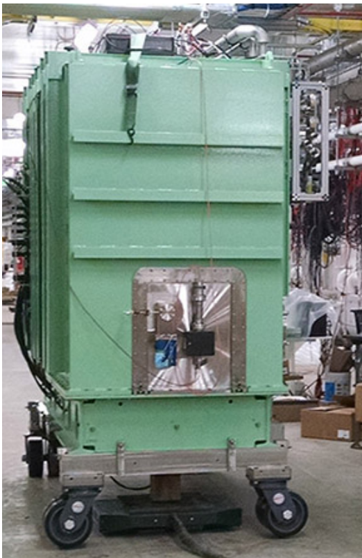
The first FRIB superconducting cryomodule was installed on FRIB's linear accelerator tunnel's beamline in March.
