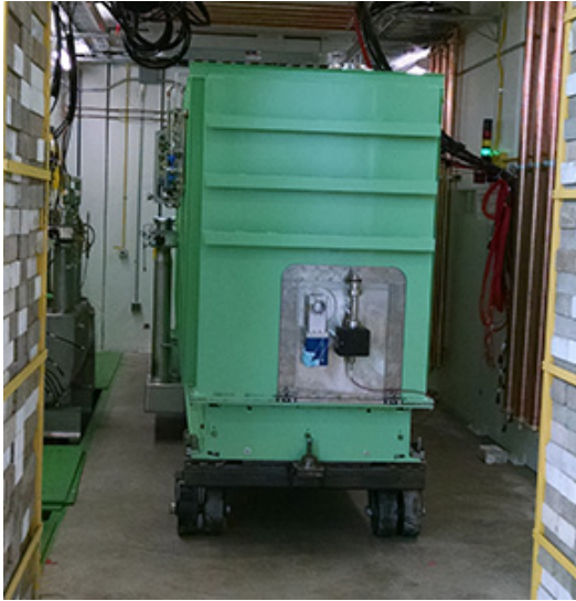
The first half-wave resonator cryomodule was successfully tested in February, enabling mass production of HWR cryomodules.
