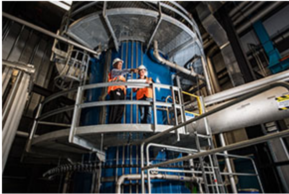
The FRIB cryogenic plant made its first liquid helium at 4.5 kelvin (K) on 16 November 2017.
