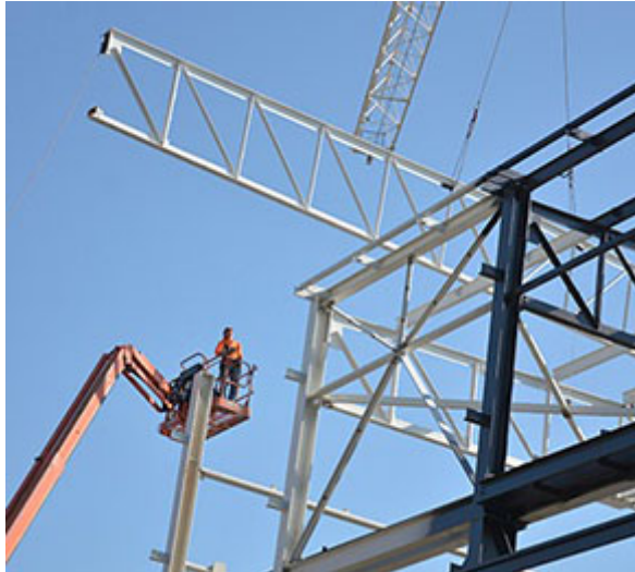
On 24 May, the last piece of structural steel on the civil-construction project was installed, marking a significant milestone.
