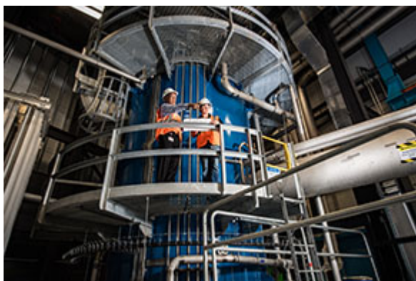
The FRIB cryogenic plant made its first liquid helium at 4.5 kelvin (K) on 16 November.
