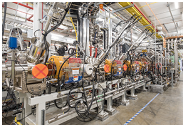
A view inside the linear accelerator tunnel at FRIB shows substantial technical progress on the accelerator beamline. (Photo credit: Kurt Stepnitz, Communications and Brand Strategy)
