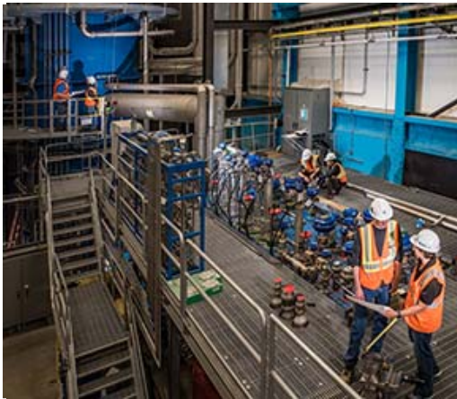
The FRIB cryogenic plant was completed in December 2017. It is now operational, and is on track to operate in 2018.
