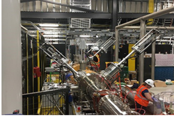
Engineers and technicians work to install beam instrumentation on the FRIB Lower Energy Beam Transport (LEBT) line.
