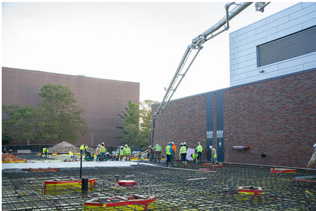
Construction continues on the MSU-funded Cryogenic Assembly Building (CAB) at FRIB. The first CAB concrete slab was placed in October.
