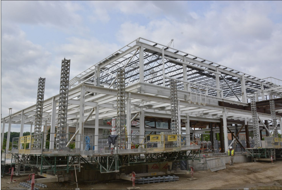
Above-ground steel placements started in April 2015, and masonry work started in June on the northeast end of the project.
