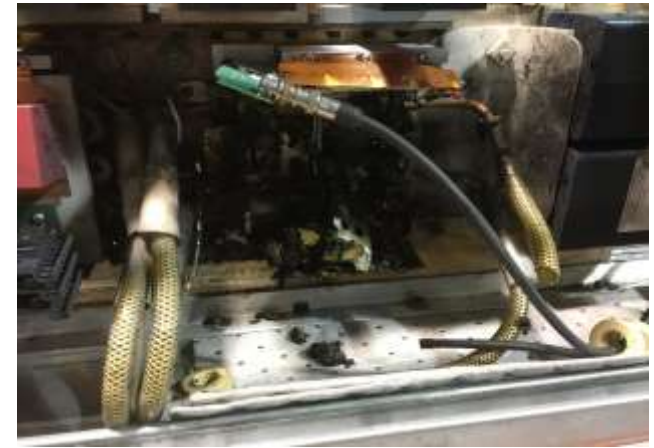
Transistor failure due to transformer saturation
